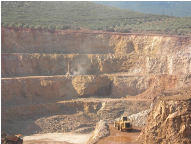
Figure 22: Modern open-pit mining of iron-nickel laterite employing sophisticated blasting technology, large haulage trucks and Doppler radar systems to monitor slope stability, Agios Ioannis mines at Neo Kokkino, Larymna, Greece. Photo: A. Demetriades
